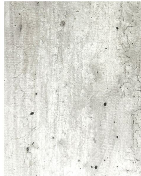
NPB 3789 Cracked Cement Light
